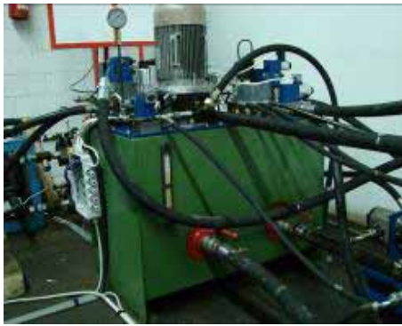
Fig. 5. The group of hydraulic tank.
