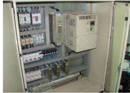
Fig. 8. The electric and electronic equipment.
