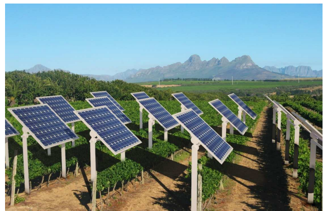
Fig. 10. Solar panels over vineyards.
