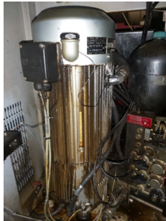
Fig. 5. Indicative heat flow sensor mounted in Emco Maxxturn 65 (hydraulic system).
