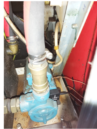
Fig. 6. Vibration sensor mounted on the cooling system pump.
