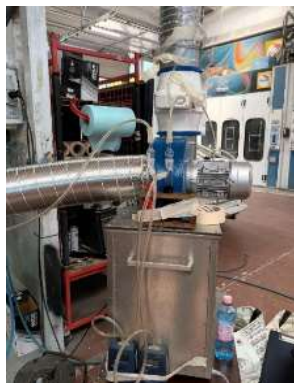
Fig. 6. Location of the filtration system.
