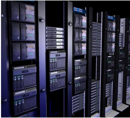
Fig. 8. Data Center general view.
