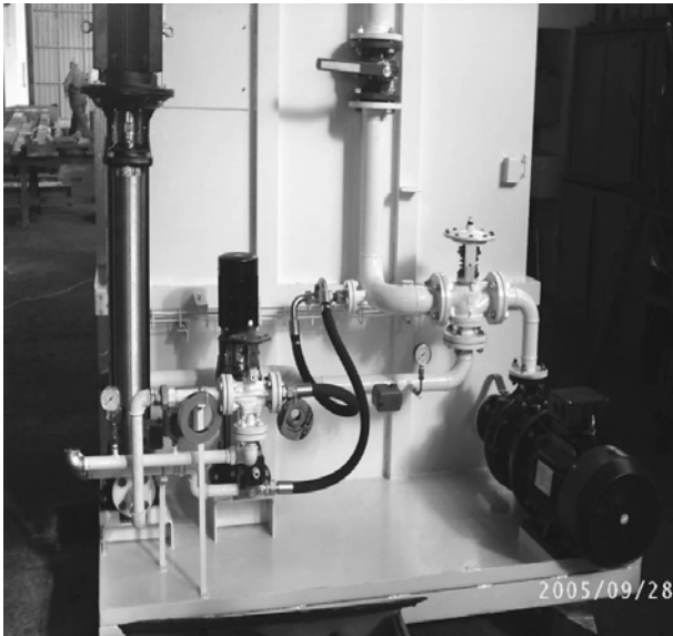
Fig. 6. The realisation of the installation, according to the schema of the cooling installation.
